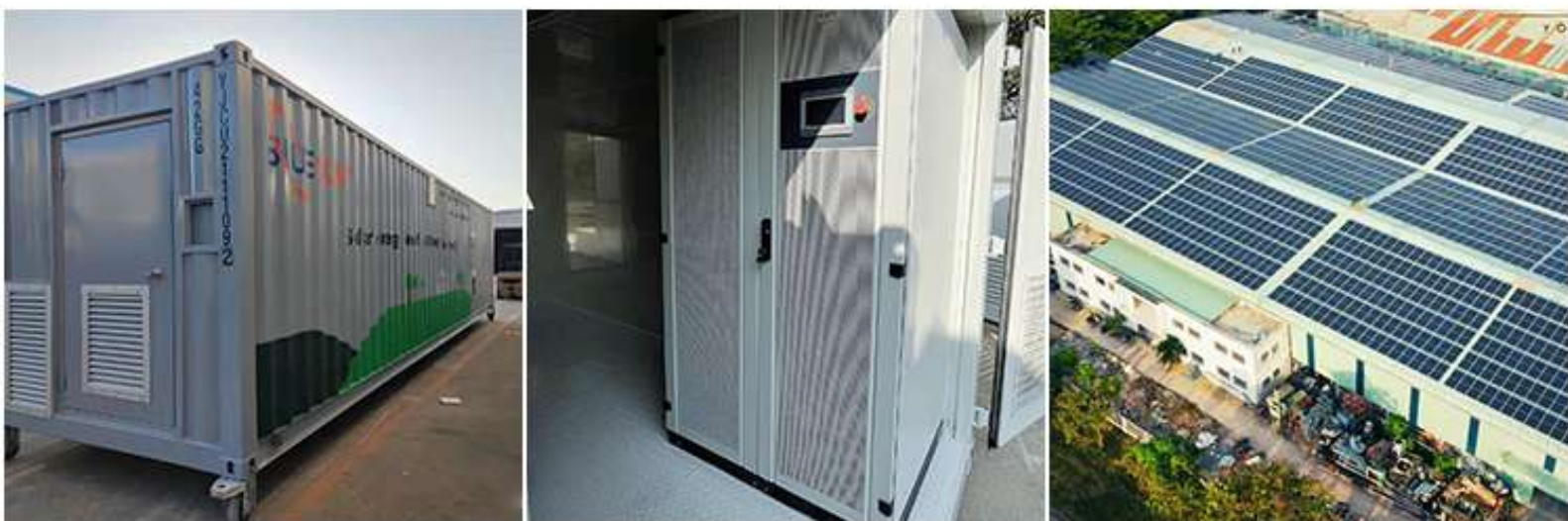
Roof energy storage system 3MW
